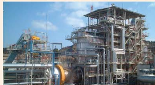
Valuable metals recycling facility
